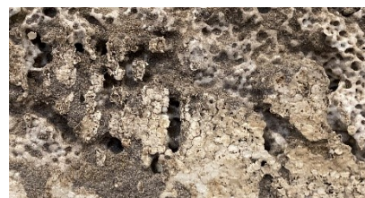
Myreskade i EPS.
