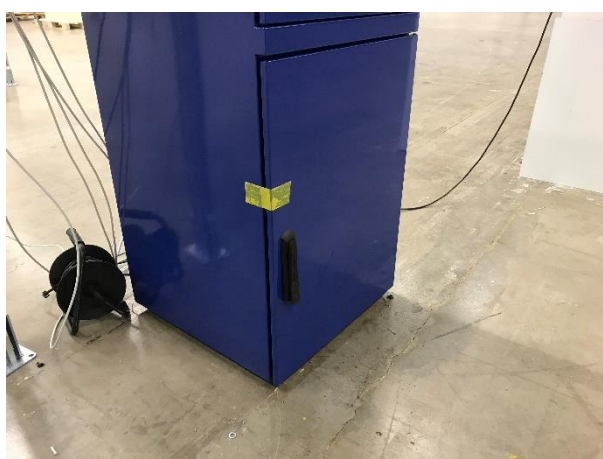
Figure 9 Sealing of cabinet for PC.
