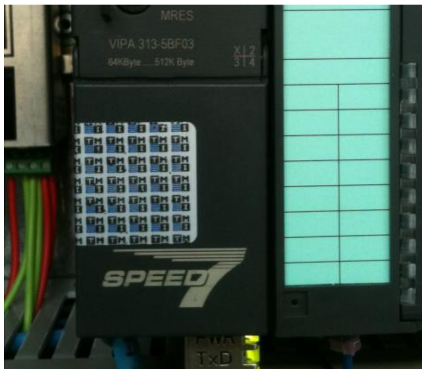
Figure 8. Sealing of access to communication terminals of the VIPA PLC
