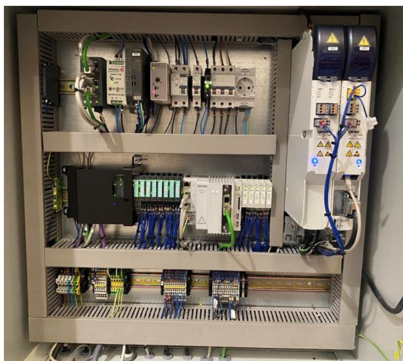
Figure 4. Control rack of ILERPES iLOC.
