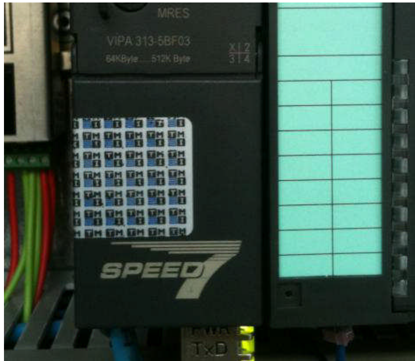
Figure 8. Sealing of access to communication terminals of the PLC
