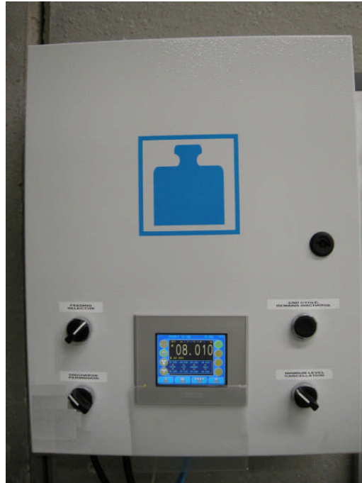
Figure 1: Control rack with operator's panel on front and weighing transducer and PLC inside
