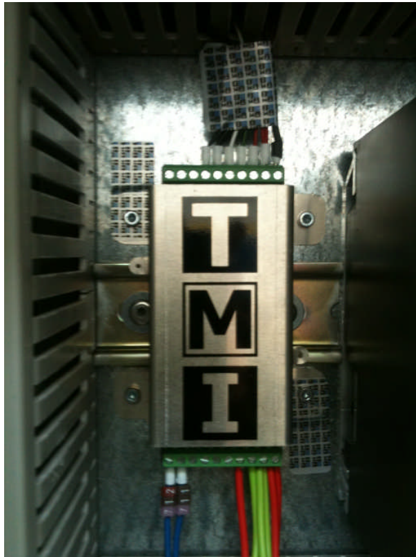
Figure 6. Sealing of LDU 78.1 weighing transducer, against removal and its load cell cable,
